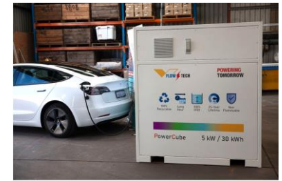
Two trial projects to support electric vehicle charging in South Korea and Australia 30 kWh/5 kW
